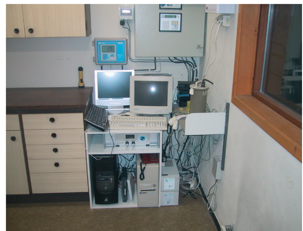
Typical NNSN indoor installation of a station
